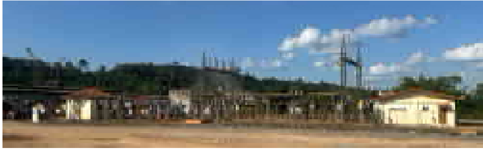
Figure 14-4: Main Transformer Station
